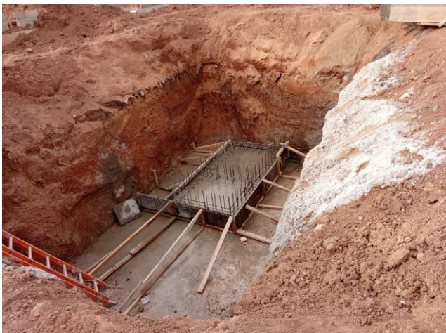
Lamashegu Septic tank.
